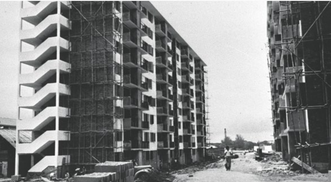
Construction of the first phase of the Bukit Ho Swee housing estate, 1961. This phase comprised five blocks of emergency flats for the fire victims.
